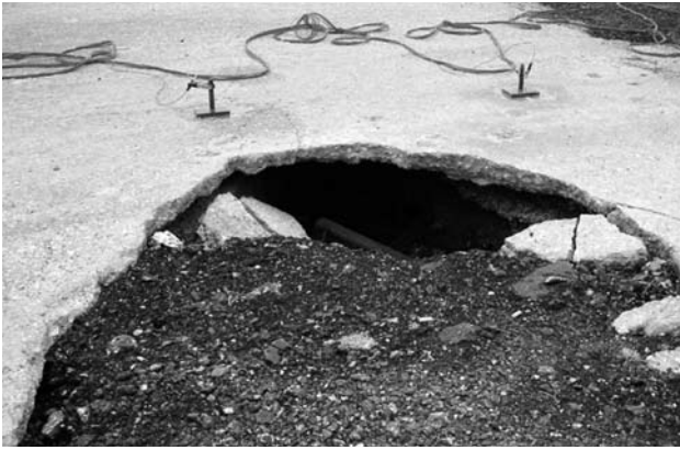
FIGURE 8 Surface exposure of an air-filled void under the concrete pavement.
